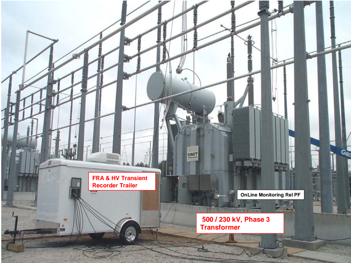
On-line FRA & Transient Recording Equipment Location Figure 3
